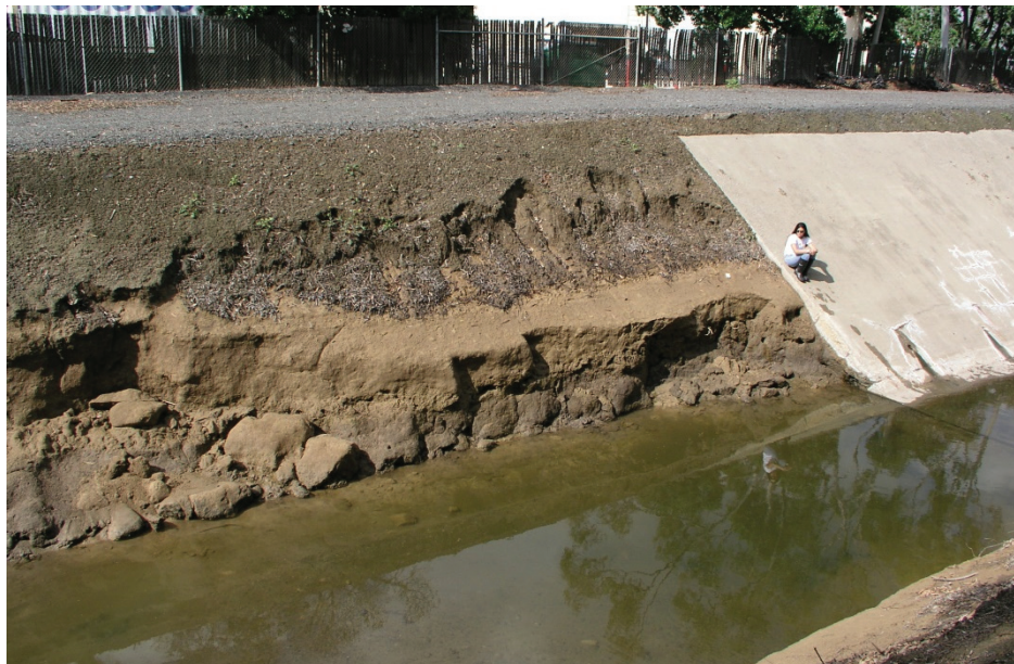
Figure 1. Erosion of unlined channel below a lined section of Barranca Channel, San Diego Creek Watershed, California (photo credit, Henry Jones).
